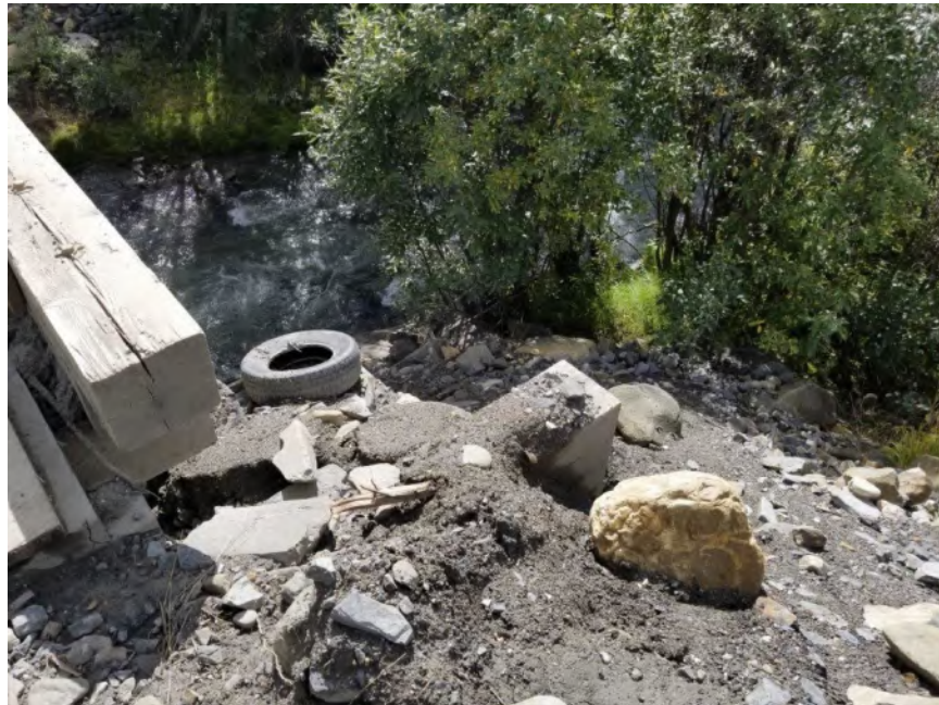
Photo 5 - Bellekeno Haul Road, Approach Erosion (August 08/20)
