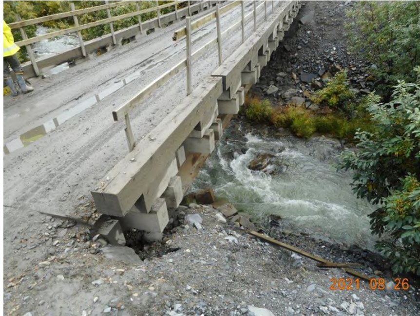
Photo 5: Bellekeno Haul Road, Approach Erosion (August 26/21)
