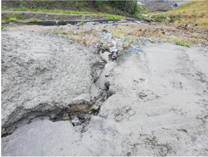
Photo 11: DSTF Tailings Erosion (August 26/21)
