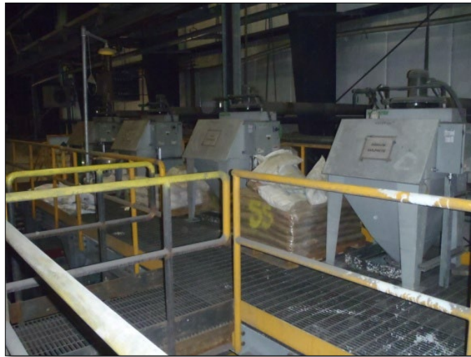
Photo 7-7: Reagent Mixing Station
