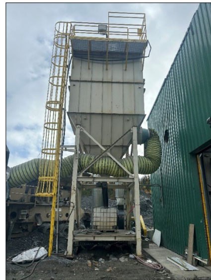
Photo 3-3: Dust Collection and Ventilation System
