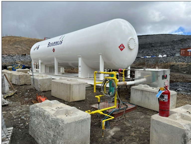
Photo 3-11: Mill Propane Storage Tank
