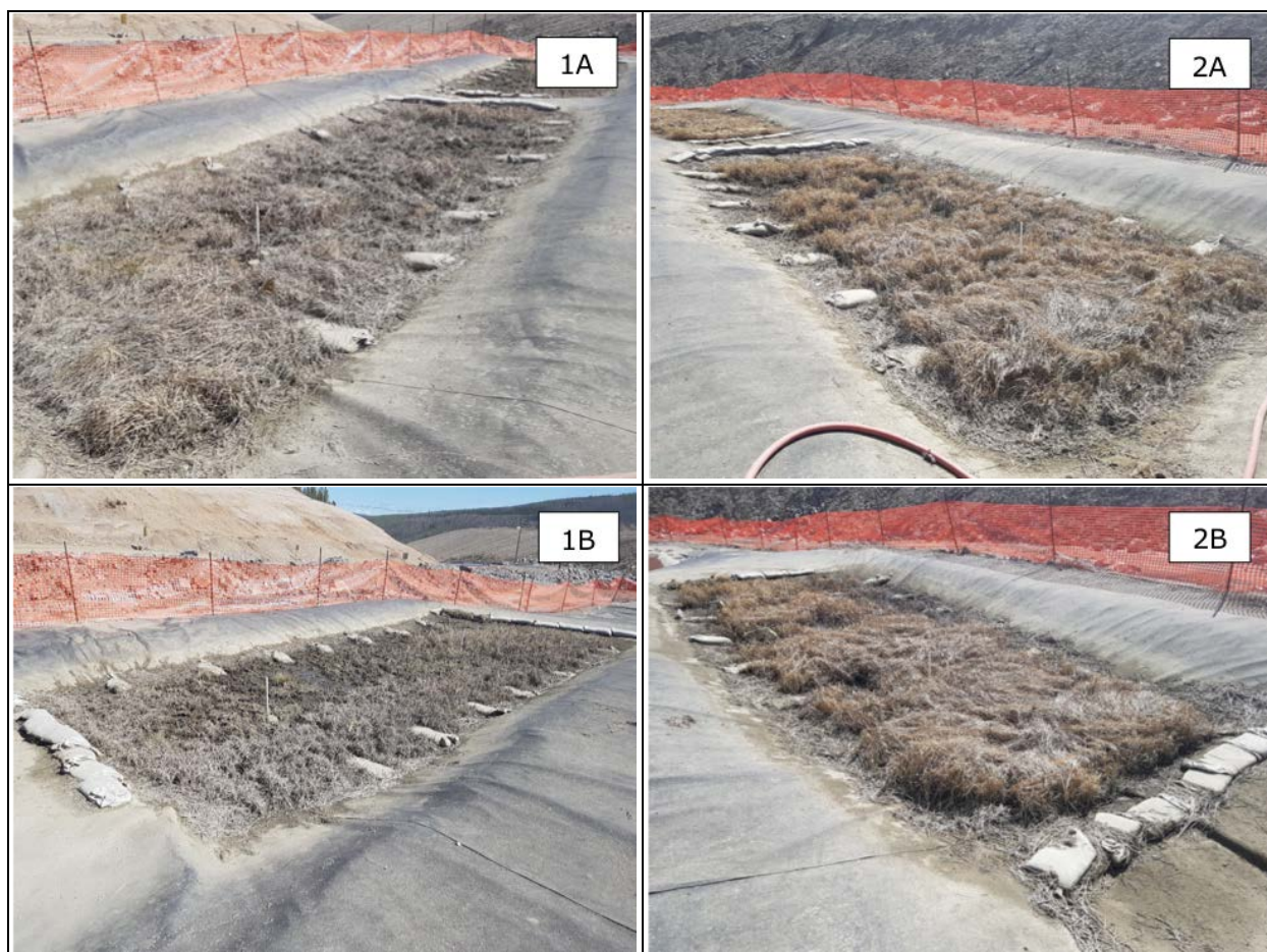
Figure 1 – Demonstration-Scale CWTS prior to start-up on May 11, 2018.
