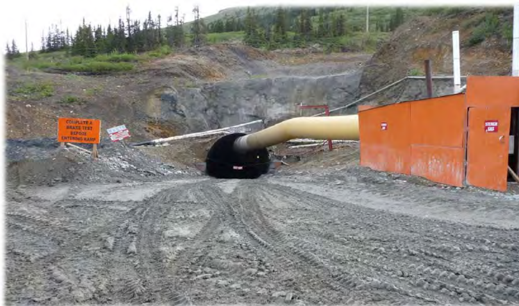
Picture 3-3: Mine Adit with Ventilation Fan and Tubing Entering Main Ramp
