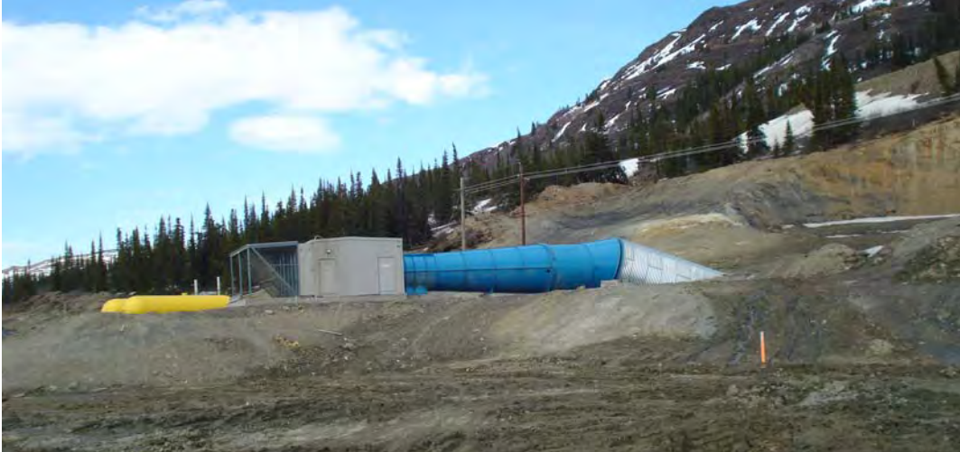
Picture 3-4: Mine Heater Fan House and Ventilation Raise
